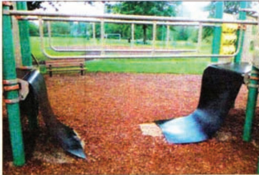
Vandals recently destroyed a rubber playground bridge at Commonwealth Lake Park. The Tualatin Hills Park & Recreation District believes the bridge was cut through with a knife.
